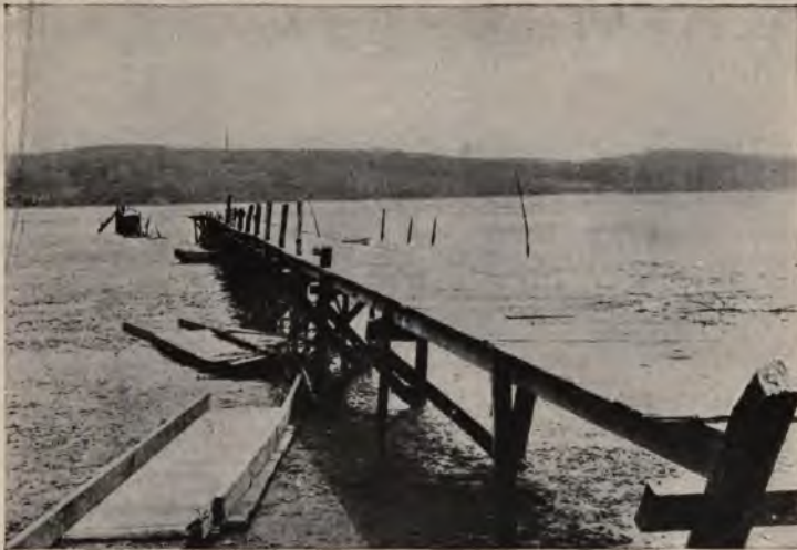
A. END OF A PIER AT INVERNESS (TOMALES BAY), CALIFORNIA, WHICH WAS DISPLACED TWENTY FEET DURING THE EARTHQUAKE OF APRIL 18, 1906. (After Omori.)
